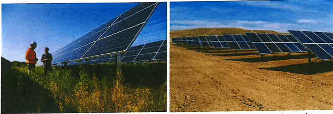
A greener way to go green—NREL Analyst Jordan Macknick and Jake Janski of Minnesota Native Landscapes survey the Aurora Solar Project's low-impact installation (left). Compare that to a traditional solar installation at Ft. Carson Army Base in Colorado Springs, Colorado (right).
